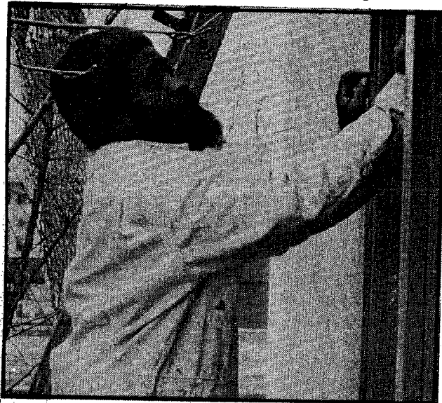
A PPL craftsman readying home for non-profit rehabilitation. Photo by Ken Meter.
