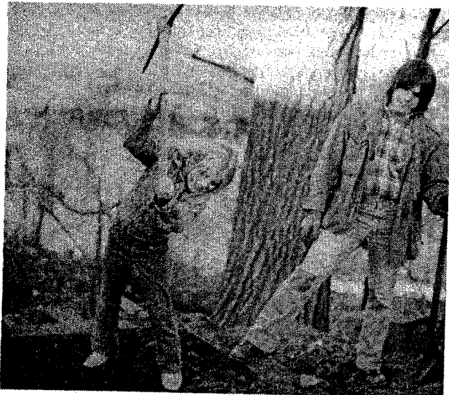
Jack Chaffee (L) and Rob Lemons work on stairway to River. Photo: Ned Pratt.
